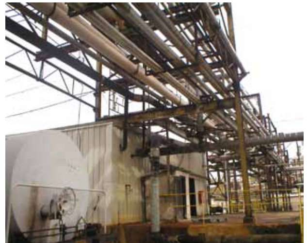
Steam tracing will keep pipes like these from freezing during cold months.
