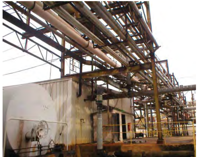
Steam tracing will keep pipes like these from freezing during cold months.
